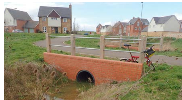
View of existing culverts and brick head walls in the flood plain
